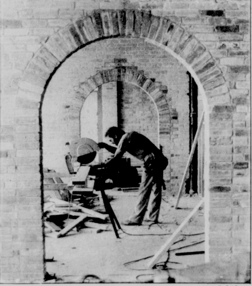
FRAMED BY A BRICK ARCH, carpenter Richard Roe works on the renovation of the Kalispell Hotel.
